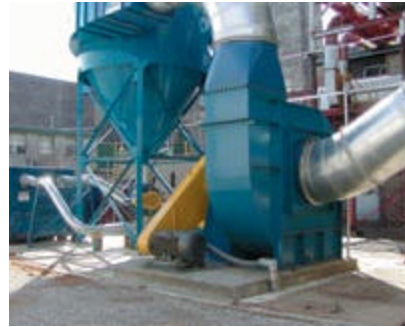
Torit 484RF dust collector from KOGER installed at Karges.
